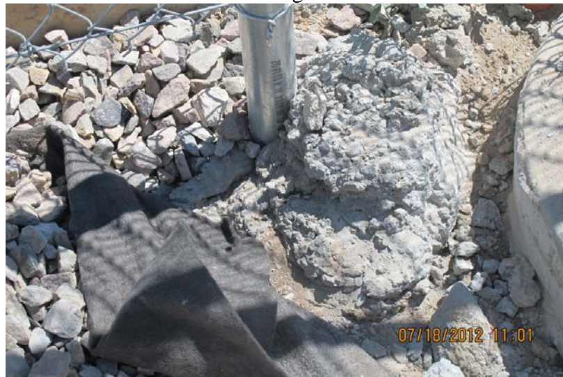
Picture 2: Lack of Water Drainage from Fence Posts
