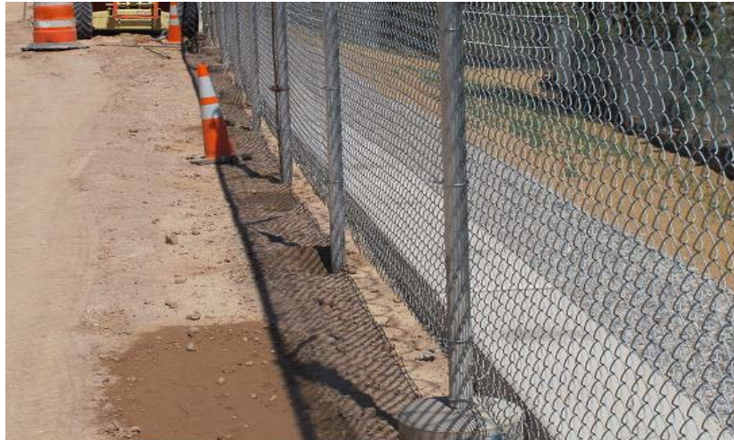
Picture 1: Pole Foundations Installed 6 Inches Below Grade
