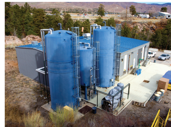
Sanitary Effluent Reclamation Facility
