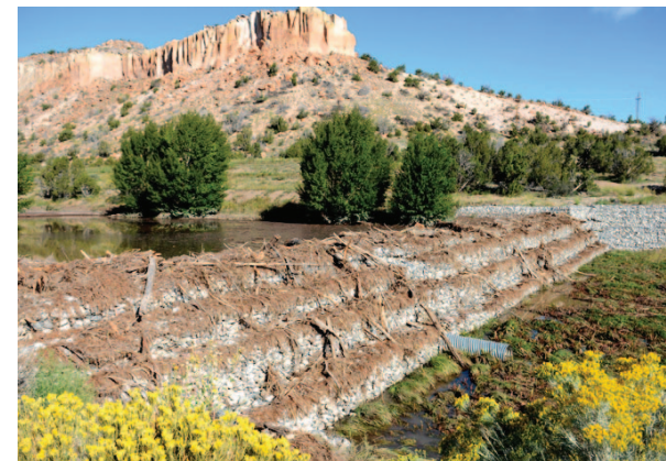
Stormwater run-off best management practice
