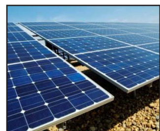
Photovoltaic Power Generation
