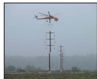
Additional 115kV Transmission Line
