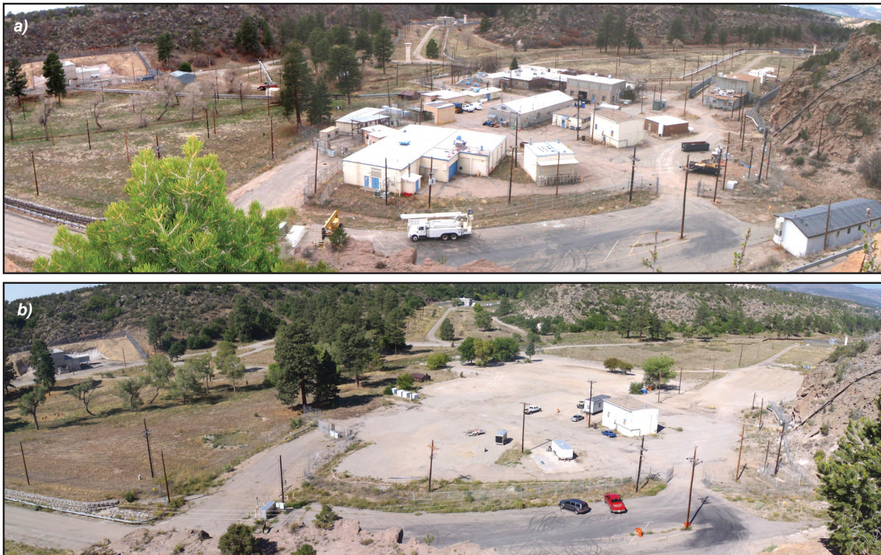
Figure 4.10: After the relocation of all Category III/IV SNM work to NNSS, the shutdown process commenced for TA-18. Panel a) depicts the site before disposition activities, while panel b) shows the site following demolition of most structures.
