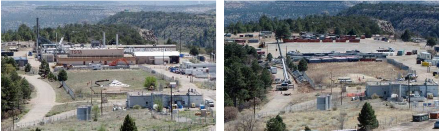
Figure 6.4: TA-21 a) before environmental cleanup as seen in May 2010, b) and after cleanup by May 2011
