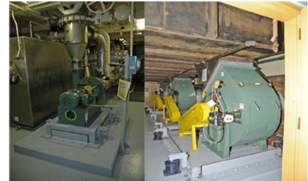
Ventilation System Equipment
