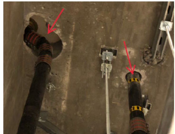
Fire Barrier Deficiencies in the Radiological Laboratory Utility Office Building
