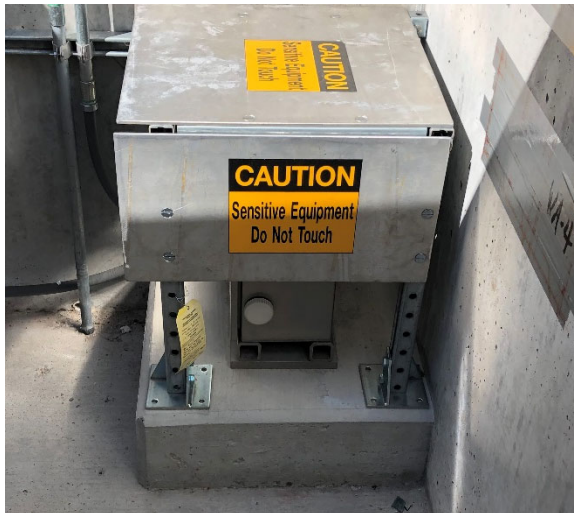
Seismic Power Cutoff Switches Redesigned and Replaced in Late 2019
