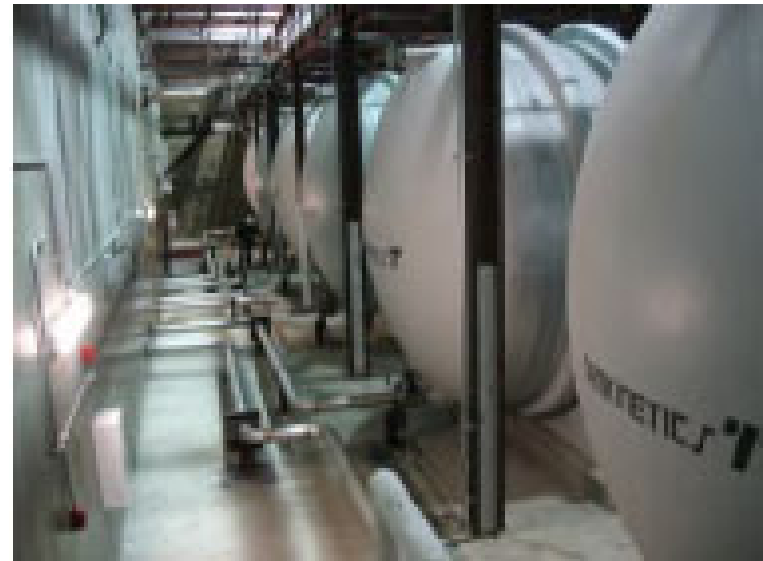
New Low-Level Influent Storage Tanks
