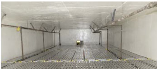
Fire Suppression System Piping
