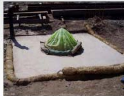
Silt saver at RLUOB storm-water discharge location for sediment control.
