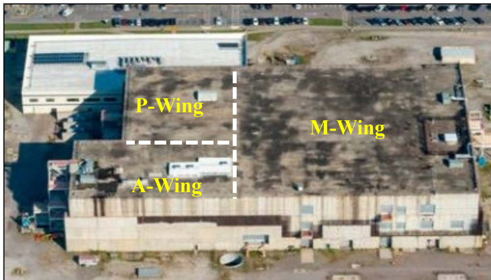
Figure 2. The three wings of Building 226-F at the Savannah River Site. A-Wing and P-Wing have non-safety recirculation ventilation systems and will house workers following an accident.
