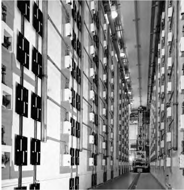
Figure 6 UK Sellafield Product and Residue Store, which became operational in 2011. Cans of plutonium are stored in separate lockers to protect against criticality accidents. Source: Sellafield Ltd.
