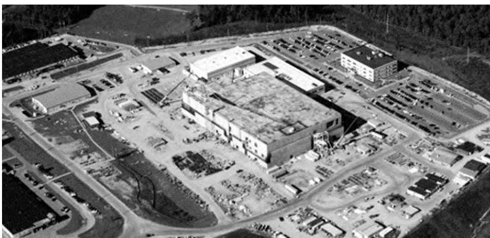
Figure 8 U.S. MOX Fuel Fabrication Facility (MFFF) under construction, 25 October 2014, at the DOE's Savannah River Site in South Carolina. Source: High Flyer, Savannah River Site Watch.
