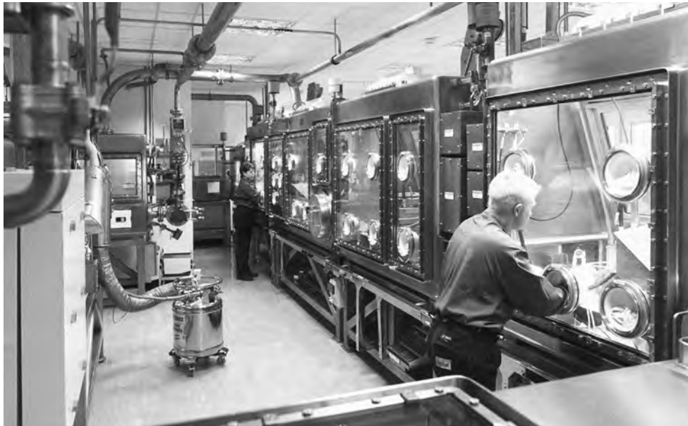
Figure 10 Glovebox line at the former Sellafield MOX Fuel Fabrication Plant. Source: UK Nuclear Decommissioning Authority.
