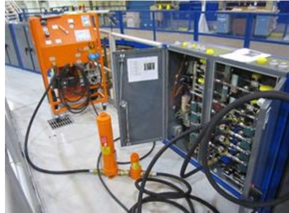
Sulfur hexafluoride reclaiming system being used on Sandia National Laboratories' Z Machine
