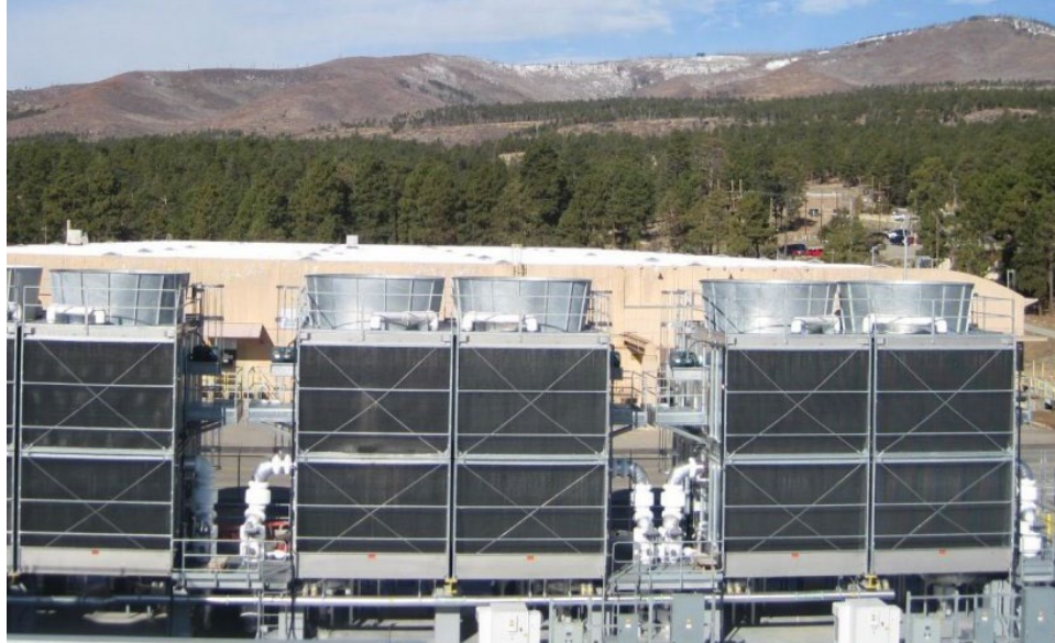
Figure A.2.2-5 Exascale Class Computer Cooling Equipment Project Cooling Towers
